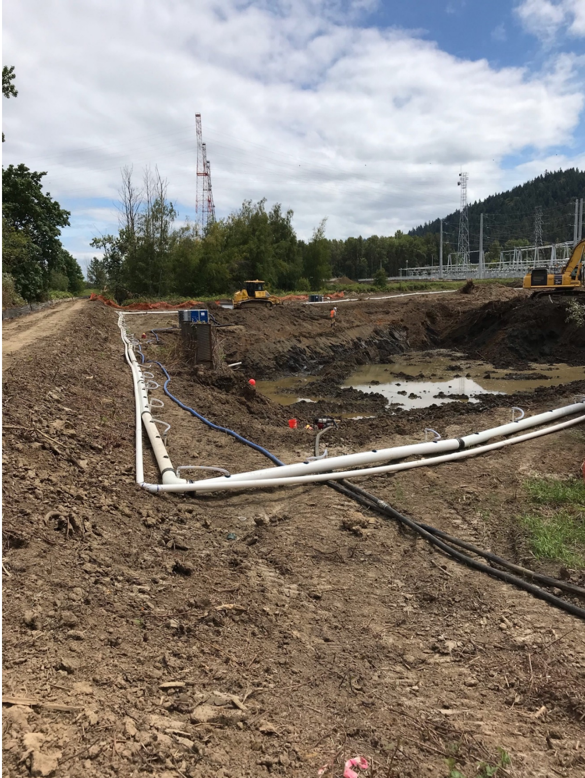
Photo 2 – Dewatering system. Shown are collection pipes (large diameter), discharge pipes (small diameter), and vacuum pump. Photo taken facing outlet of North Channel pre-breach.
