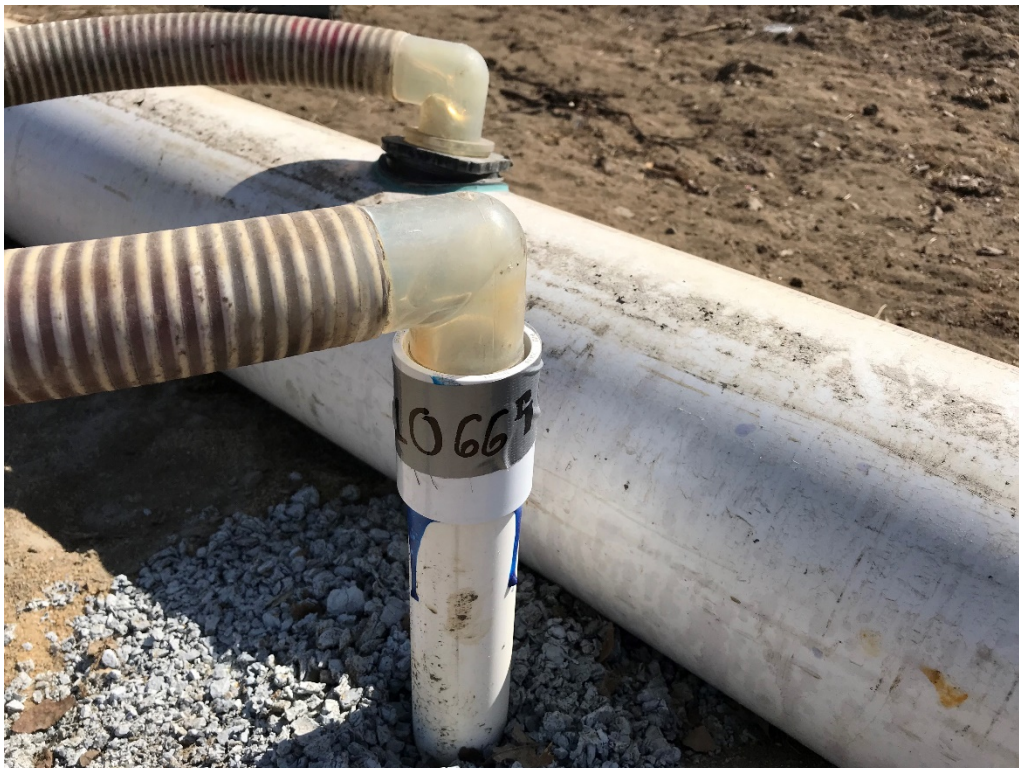
Photo 4 – Close-up of vertical dewatering pipe coupled to collection pipe. Note bentonite seal at base.
