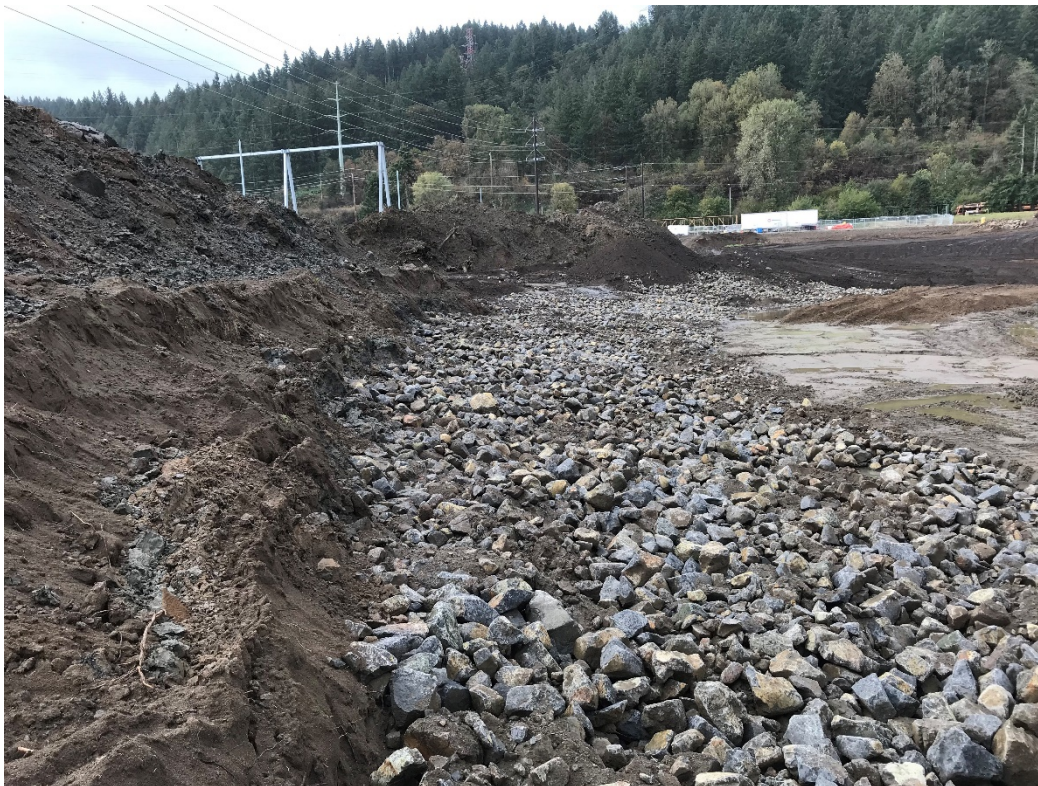
Photo 9 – Closeup of rock toe installation in Sub Area 3. Photo facing NW Marina Way.
