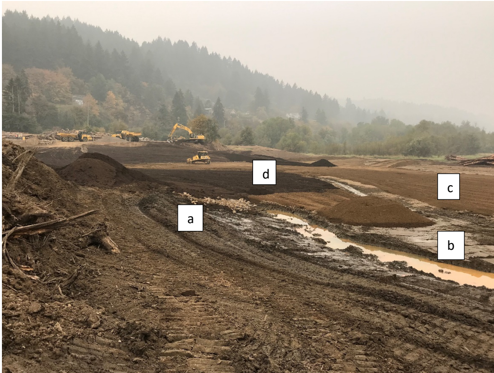
Photo 8 – a. Rock toe installation; b. exposed native soil; c. 3/4" minus gravel/topsoil mix; d. topsoil (Sept. 15, 2020)
